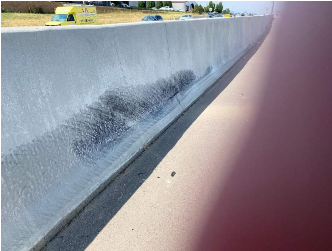
Type 7 barrier in good condition. Note tire marks and crack for repair
