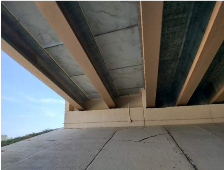
Acres Green, Slope Paving Cracking, Requires Maintenance
