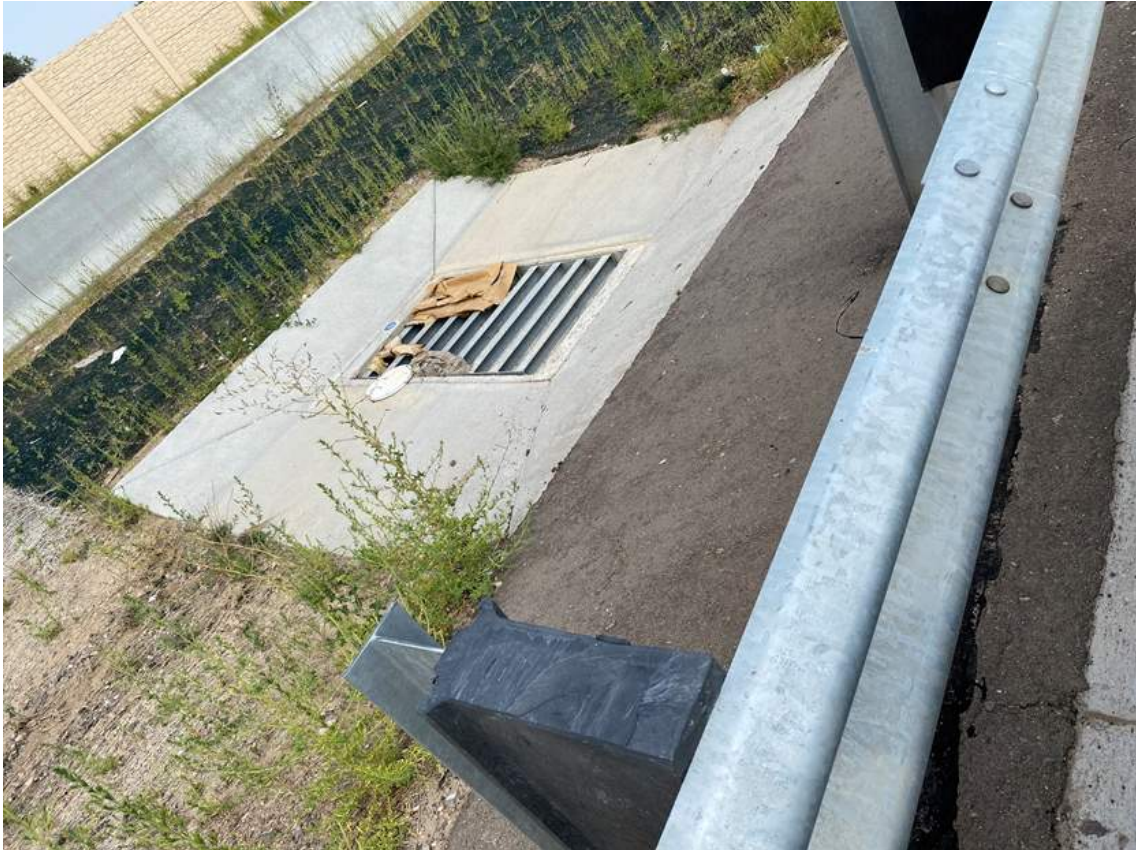
Typical Median Inlet, Requires Minor Maintenance
