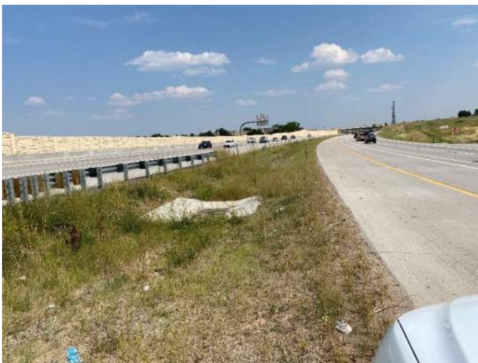
Typical Median Inlet, Generally Good Condition
