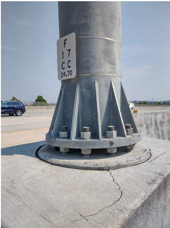
Typical Median Barrier Cracking, Requires Maintenance
