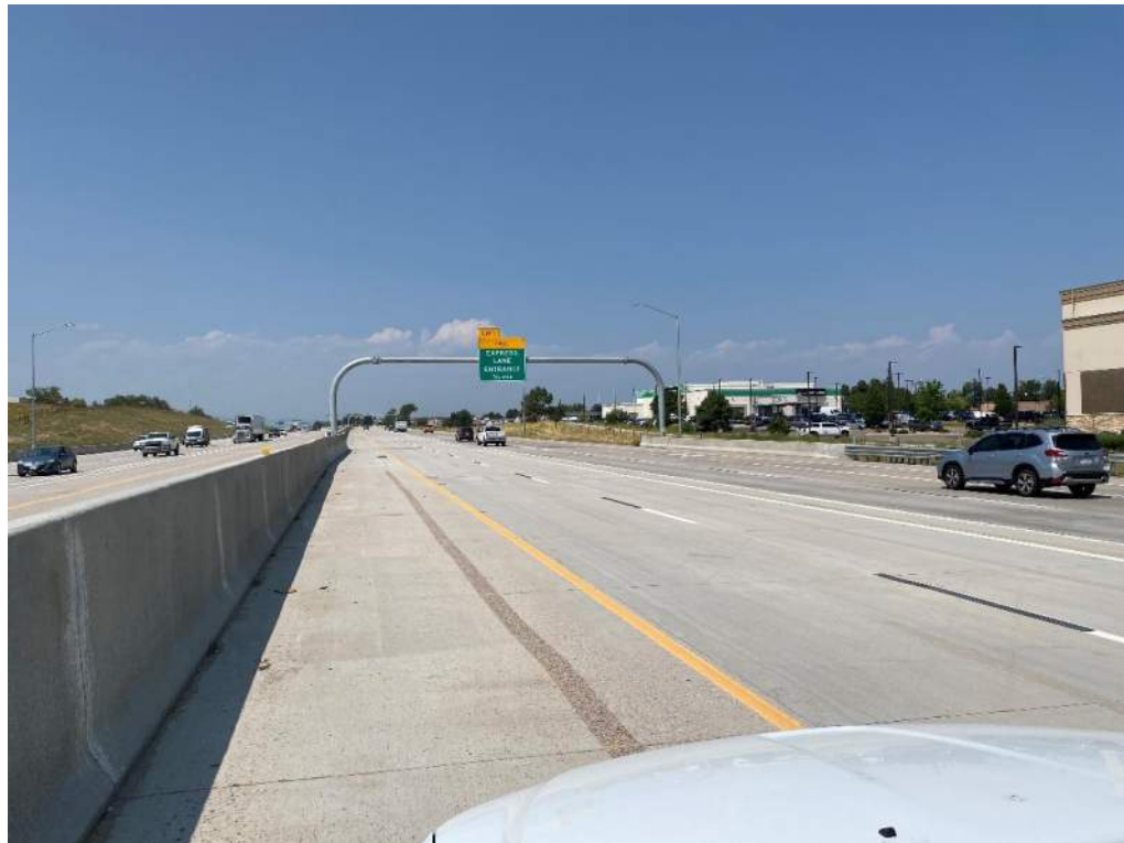
Typical Monotube sign, good condition, entrance to west bound Express Lanes
