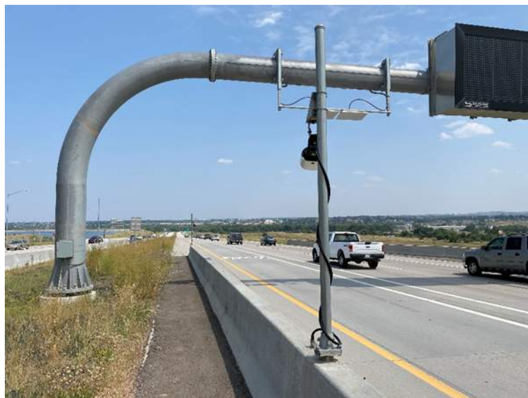
Typical Tolling Device, Good Condition
