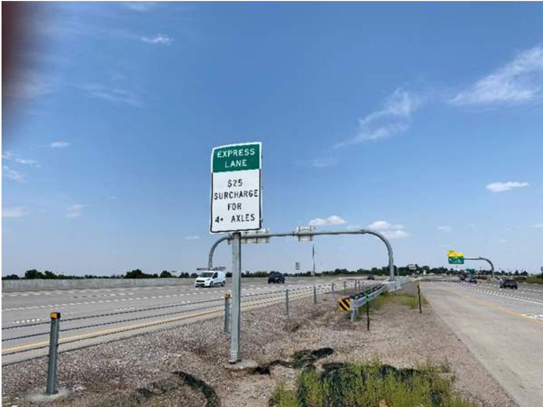
Typical Barrier Installation, Condition Good
