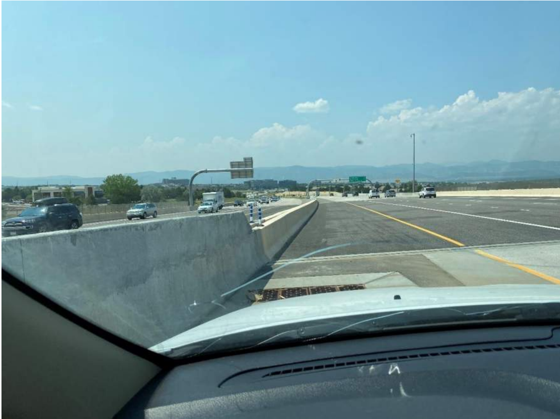
Typical Median Inlet, Good Condition with only minor sweeping and general maintenance
