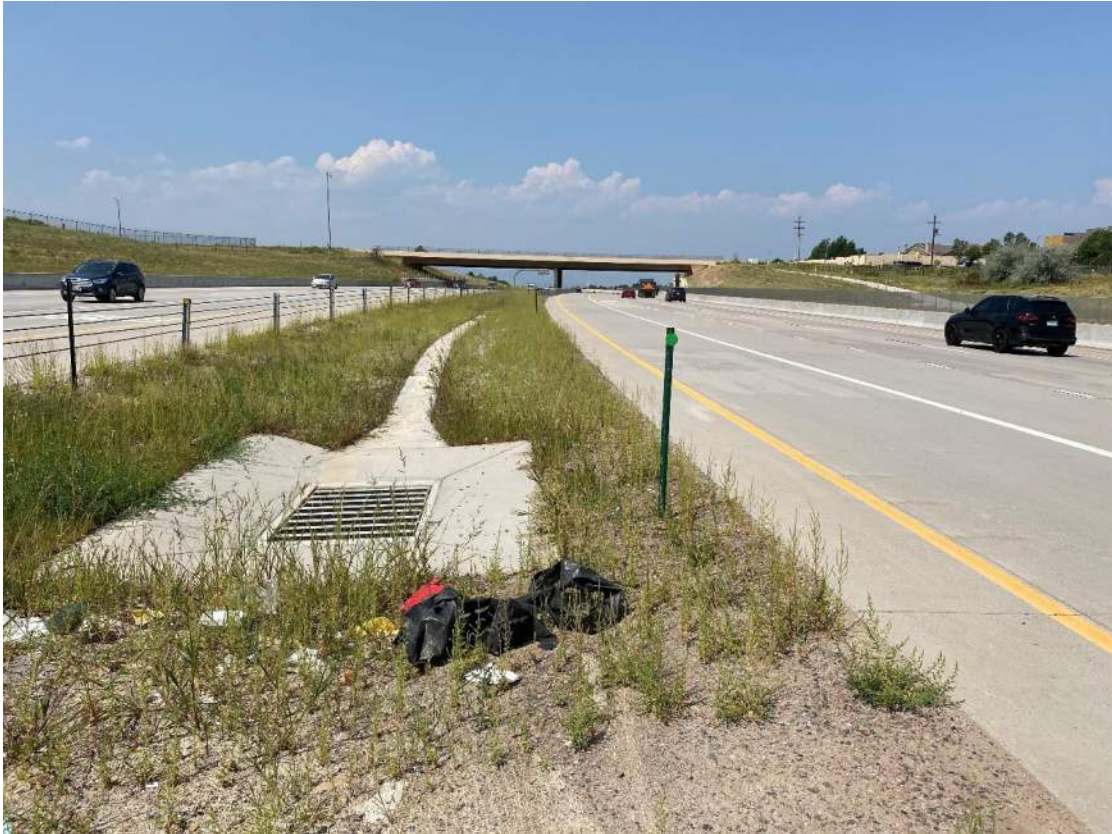
Typical Median Inlet, Requires Debris Cleanup, Inlet Good Condition
