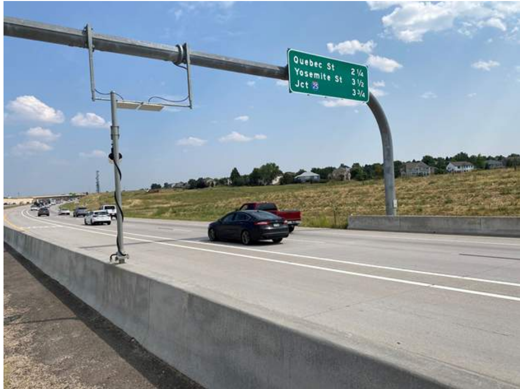
Typical Tolling Devices, Good Condition
