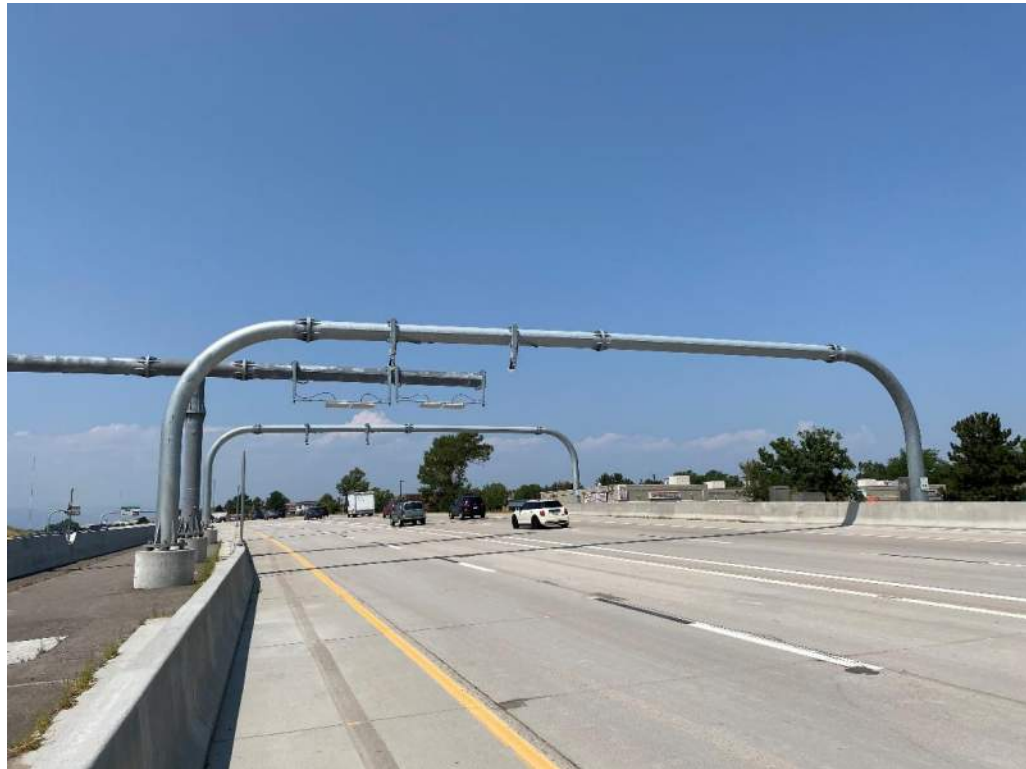
Typical Cameras and license plate devices over double express lanes, Good Condition
