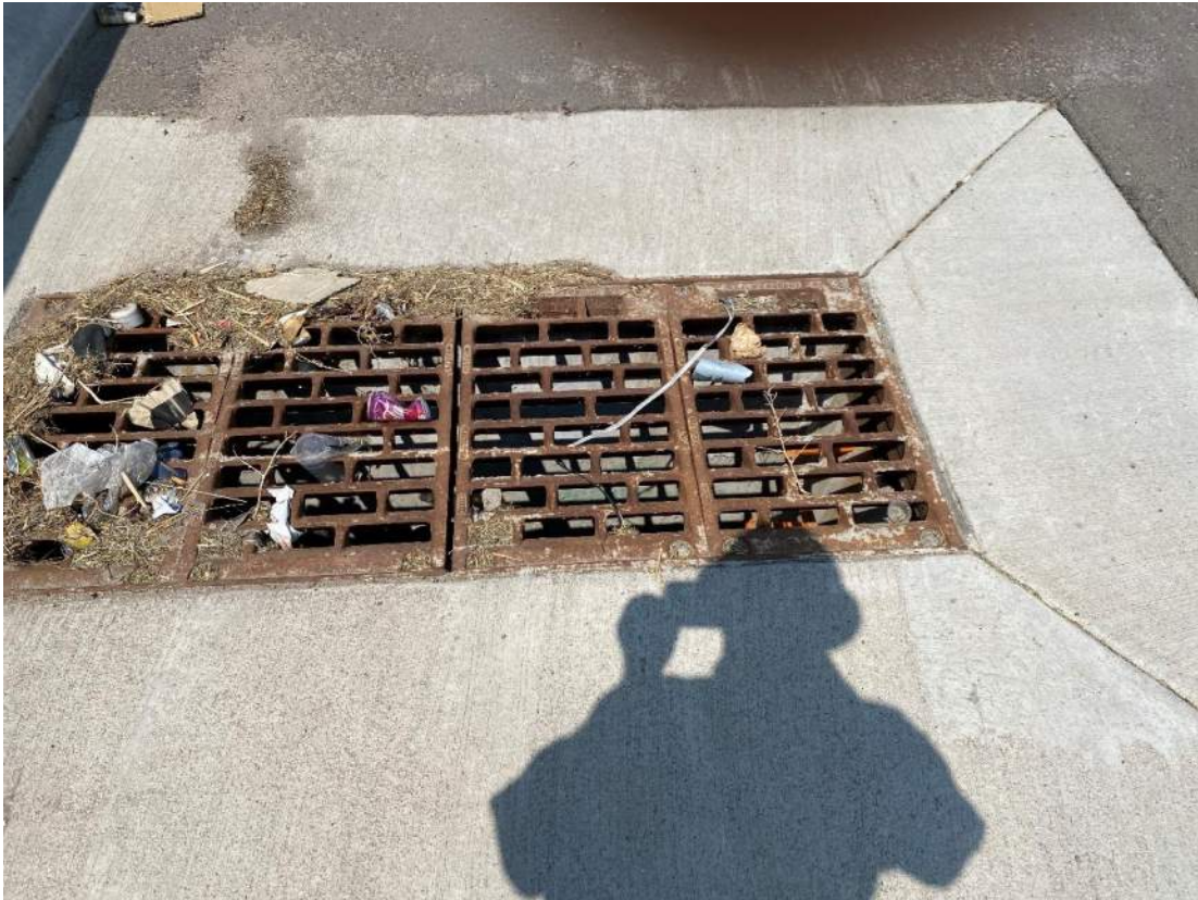
Typical Inlet and apron, Good condition, Required routine maintenance for trash and debris
