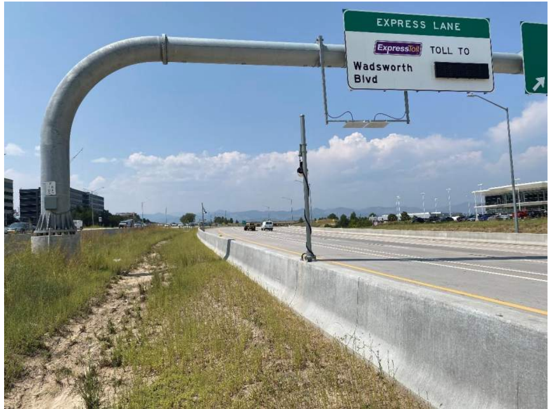
Typical Tolling Devices, Good Condition
