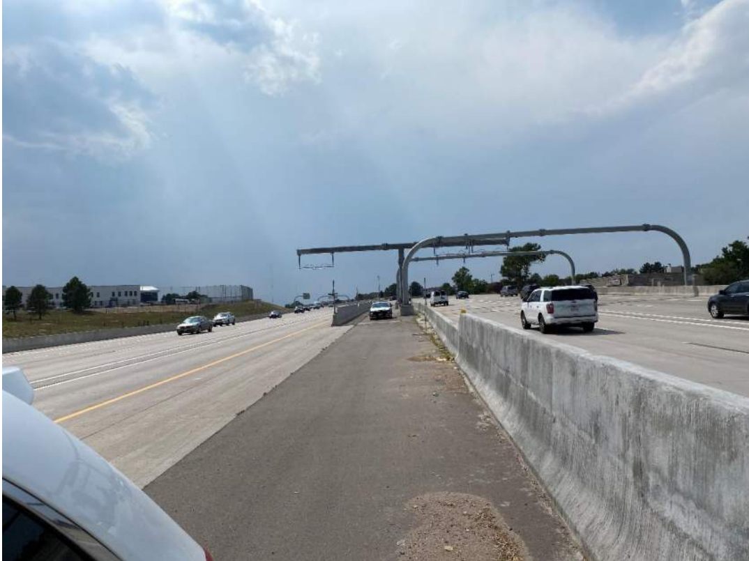
Typical Median Inlet, Requires Sweeping Sediment Removal
